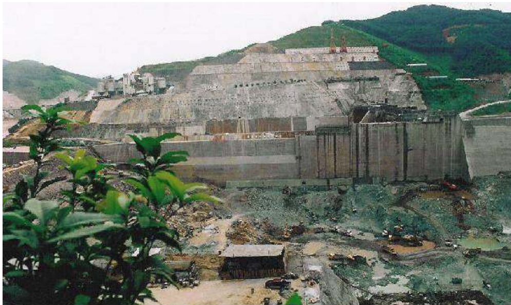
The Jinghong dam, under construction on the Lancang River. (See our Jinghong photo gallery .)
